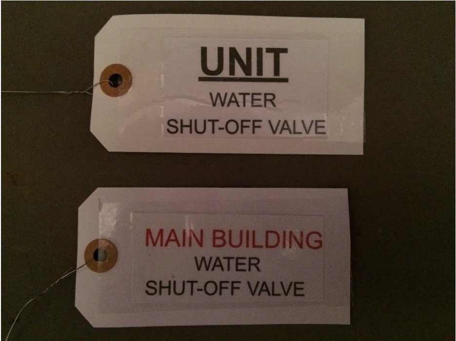
Picture 11 – Tags applied to the Master Shutoff Valve and the Unit Shutoff Valve.
