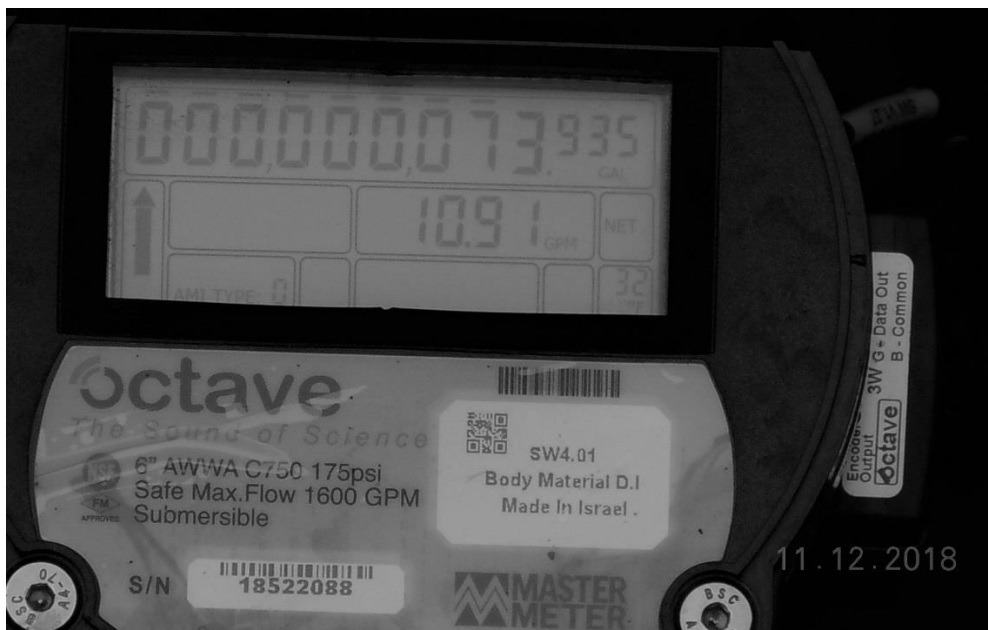
Picture 3 – New meter face.
