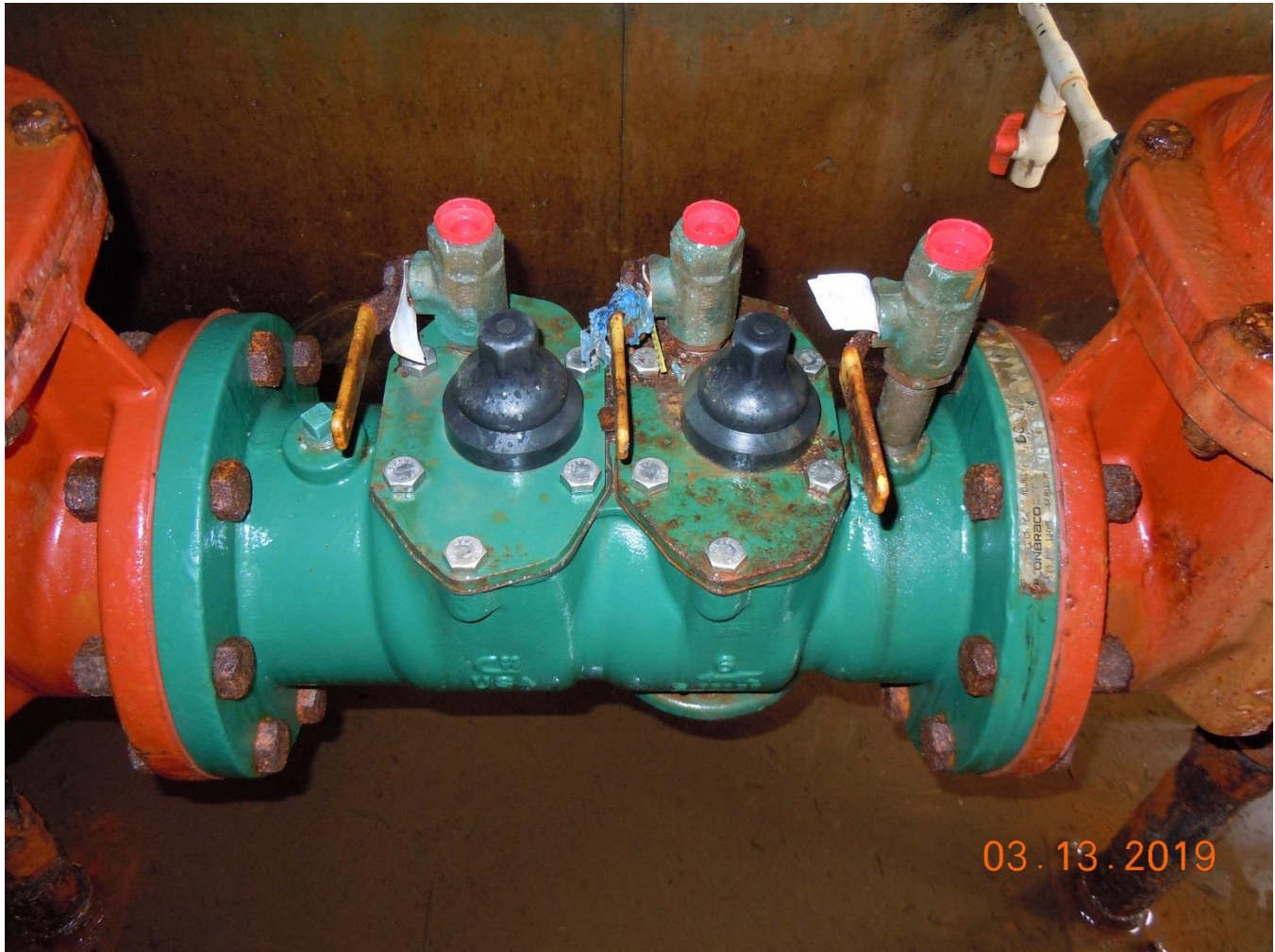
Picture 4 – Backflow Protection Apparatus.
