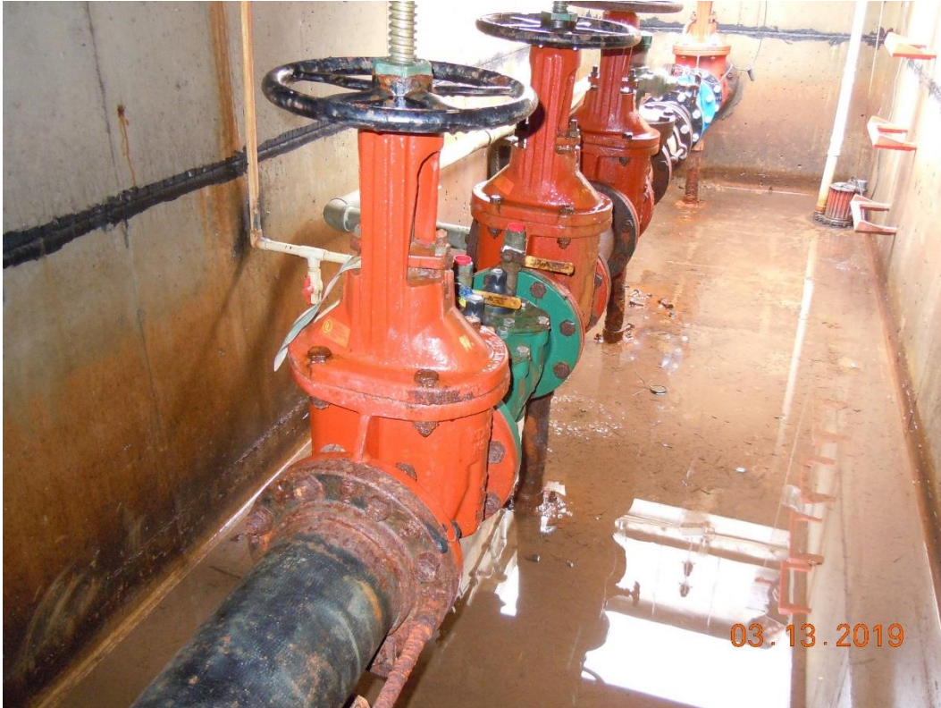
Picture 2 – The major components of the Pit are shown from the exit end looking back toward the entry end.
